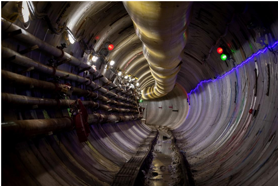
Figure 1.2: Example of an underground cable. Source: National Grid
