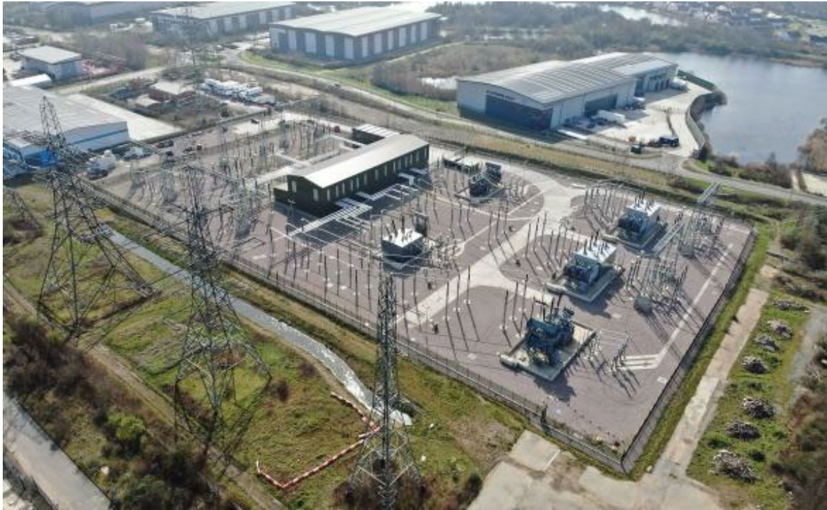
Figure 39: Example AC substation
